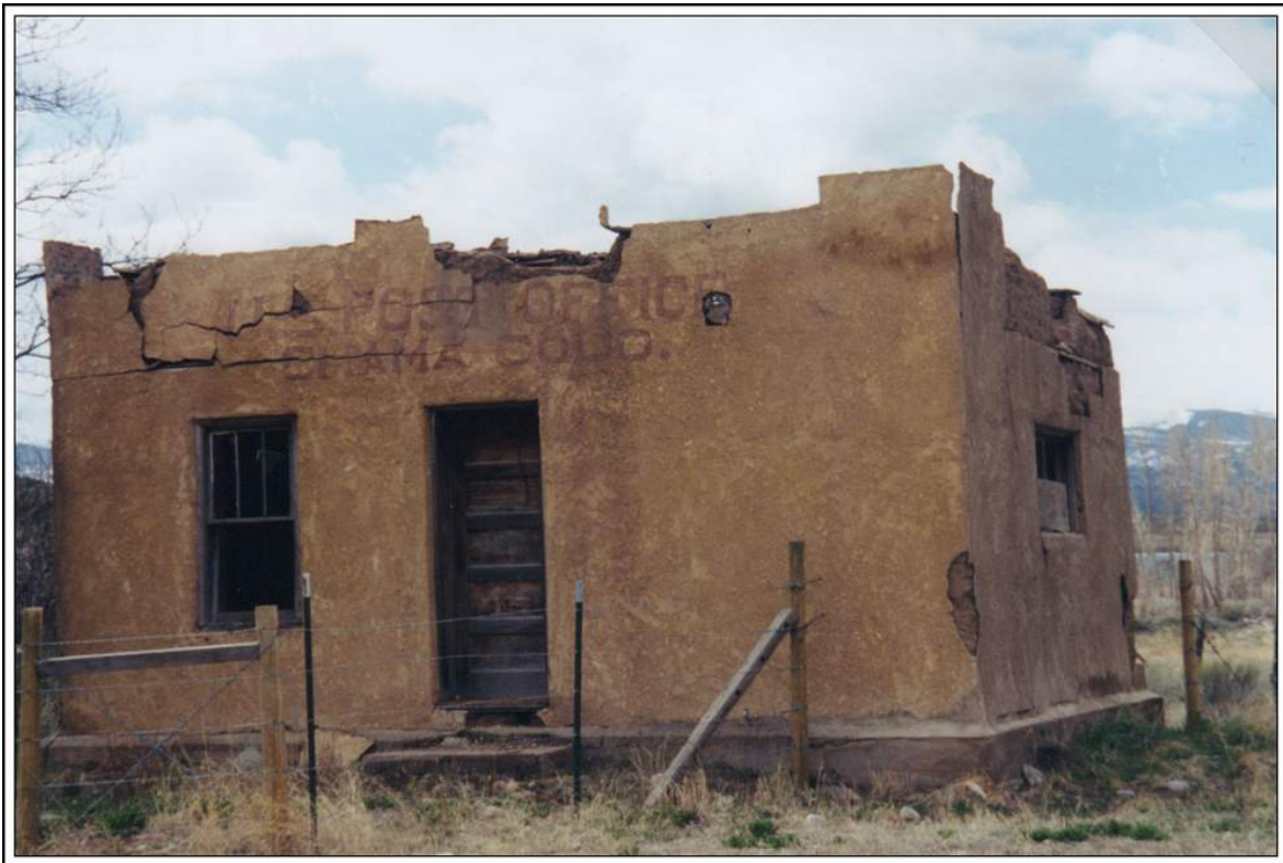
The old post office building at Chama, Colorado – The legend is faintly visible above the door. Photograph by William H. Bauer May 11, 1999
