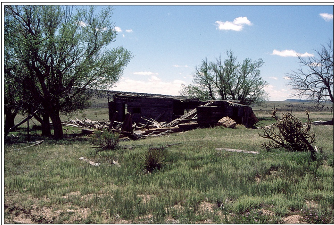
The remains of an abandoned log building at the site of Lascar, Colorado Photograph by William H. Bauer May 17, 1999
