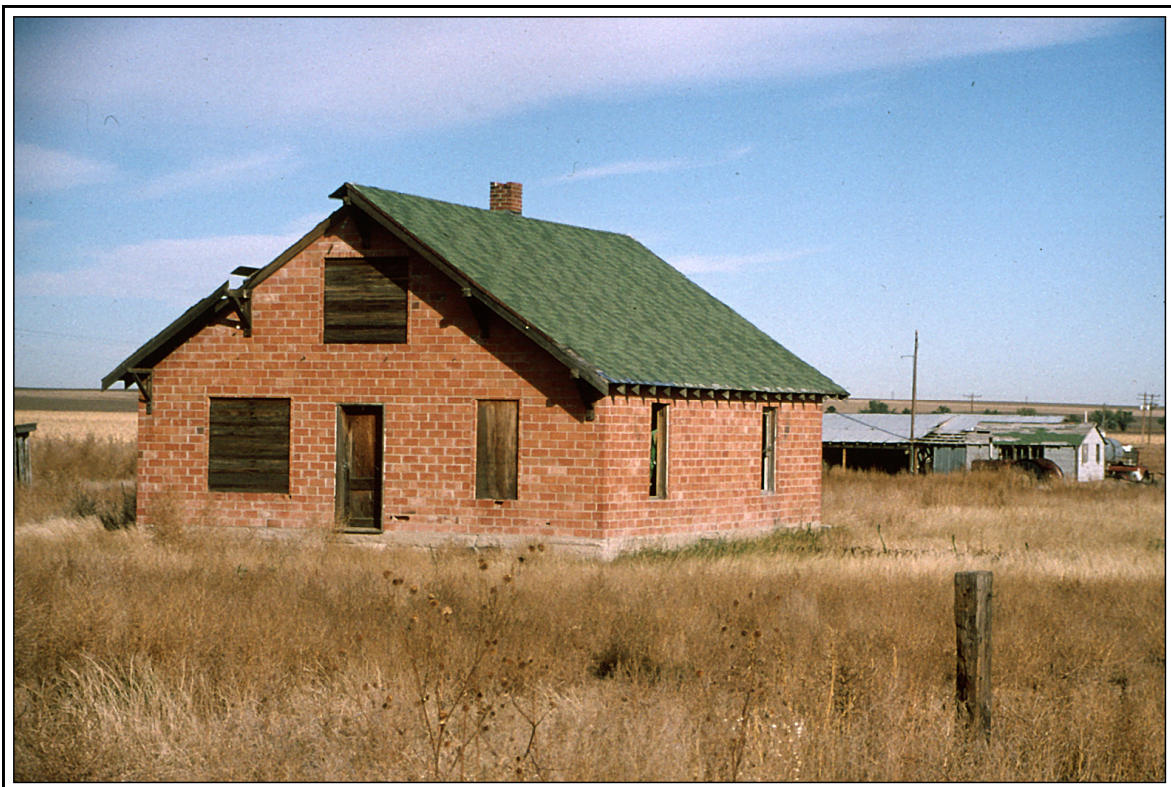
Abandoned building at the location of the Comanche, Colorado Post Office. Photograph by William H. Bauer October 15, 1997
