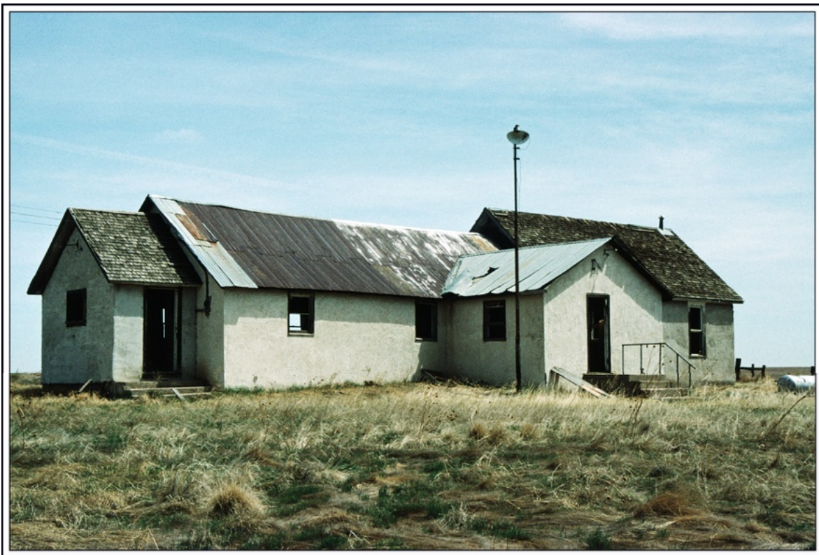
Abandoned Sand Creek Arroyo 4-H Club Building, Adena, Colorado Photograph by William H. Bauer May 14, 1996
