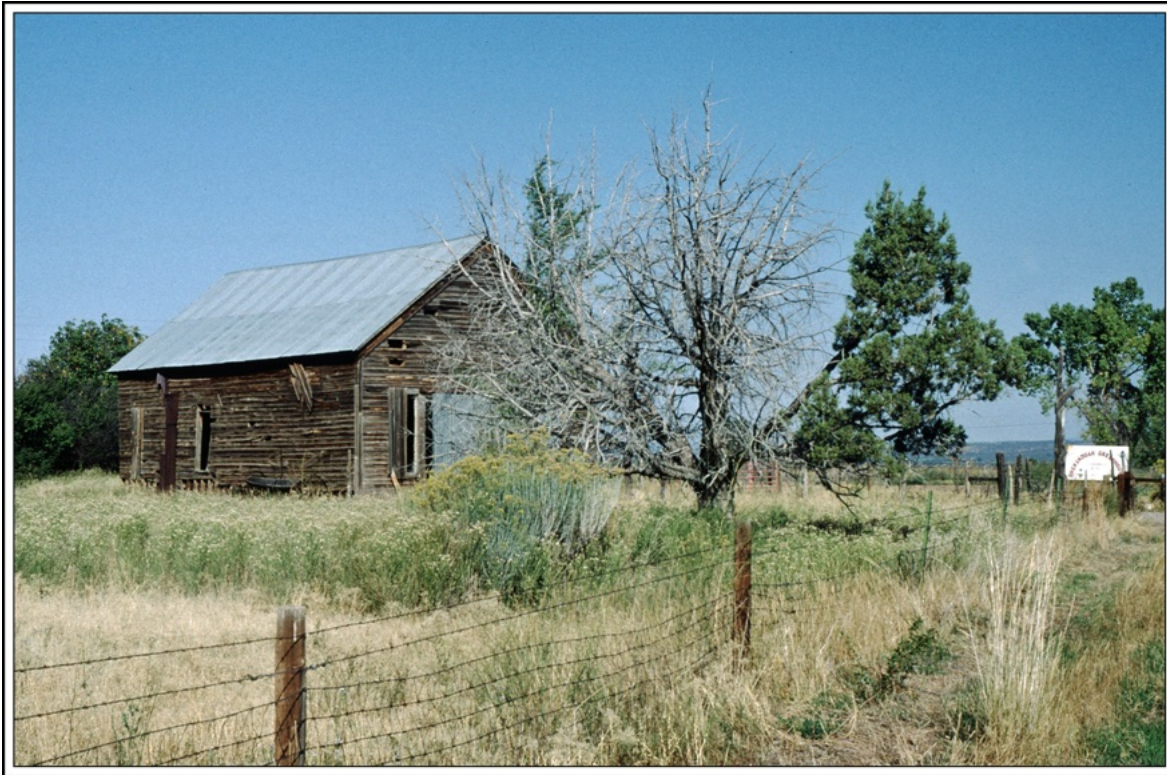
Abandoned building at the location of Shenandoah, Colorado Photograph by William H. Bauer September 22, 1994
