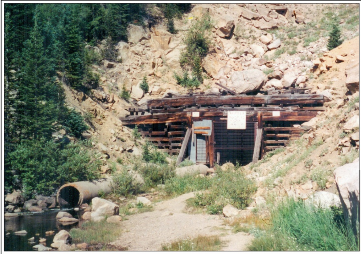
Entrance to the Busk-Ivanhoe (Carleton) Tunnel Photograph by William H. Bauer August 29, 2001
